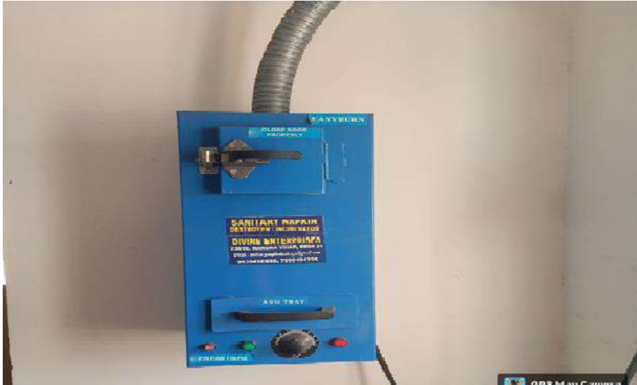
Fig.12. Sanitary napkins incinerators in women's hostel
