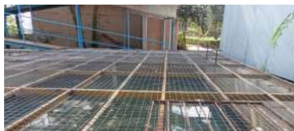
Fig. 5. Effluent treatment plant
