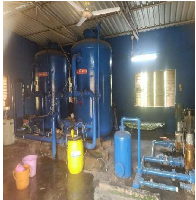
Plate 2. Water Treatment Plant in SSU
