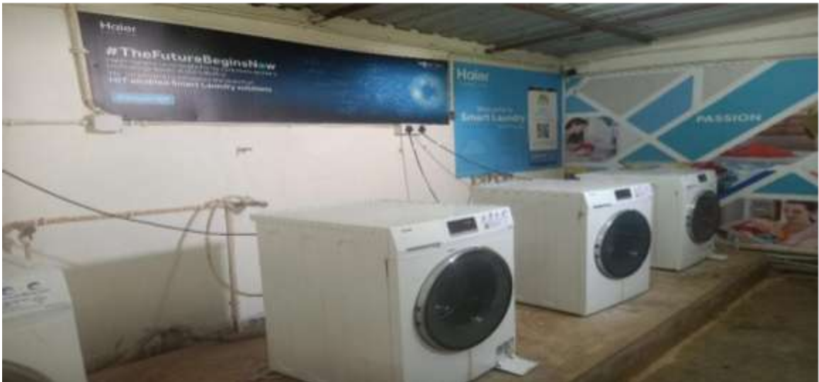
Plate 12: Water efficient appliances installed in SSU
