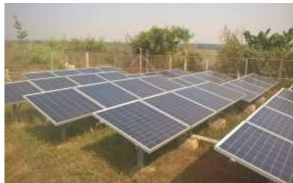
Fig. 3. Solar panels installed in the campus
