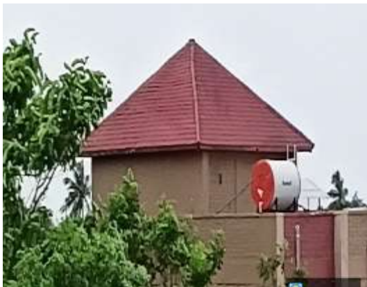
Plate 3. Solar Water Heater at rooftop
