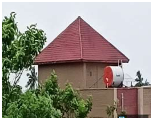
Plate 3. Solar Water Heater at rooftop
