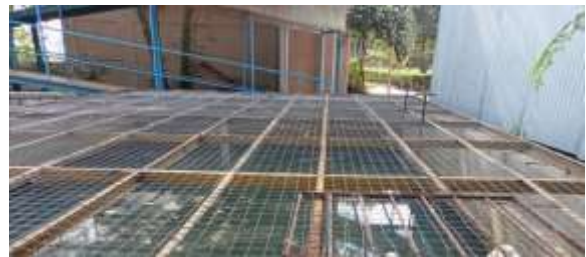
Plate 2. Effluent treatment plant
