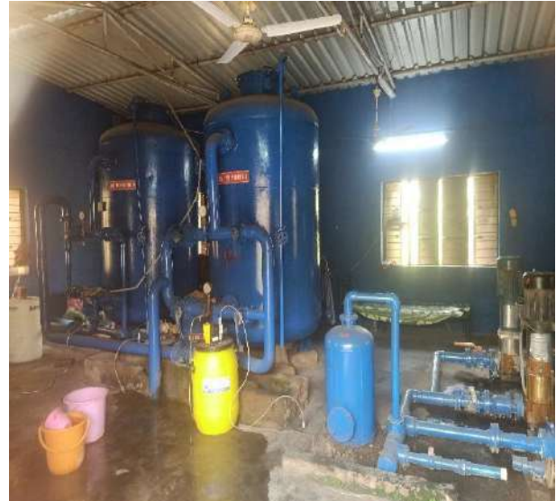
Plate 2. Water Treatment Plant in SSU
