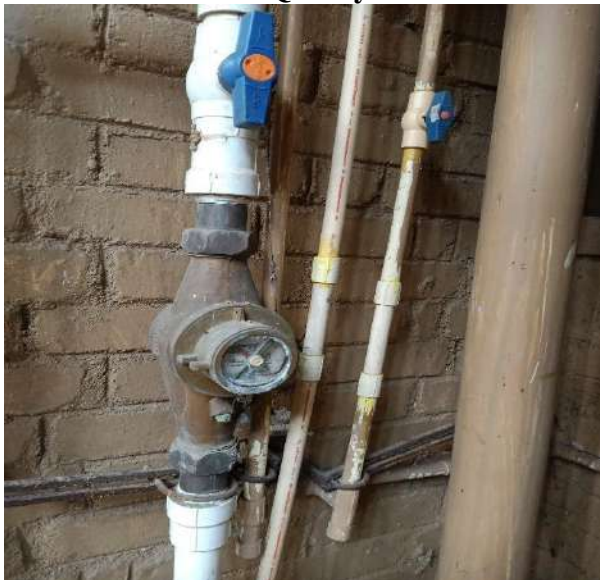
Plate 3. Water meters to track consumption
