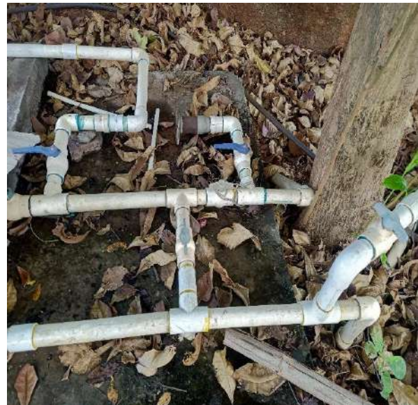
Plate 4. Water meter pipes to track consumption
