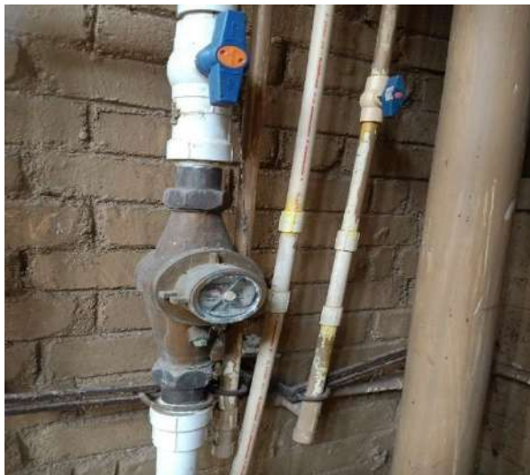
Plate 1. Water meters to track consumption
