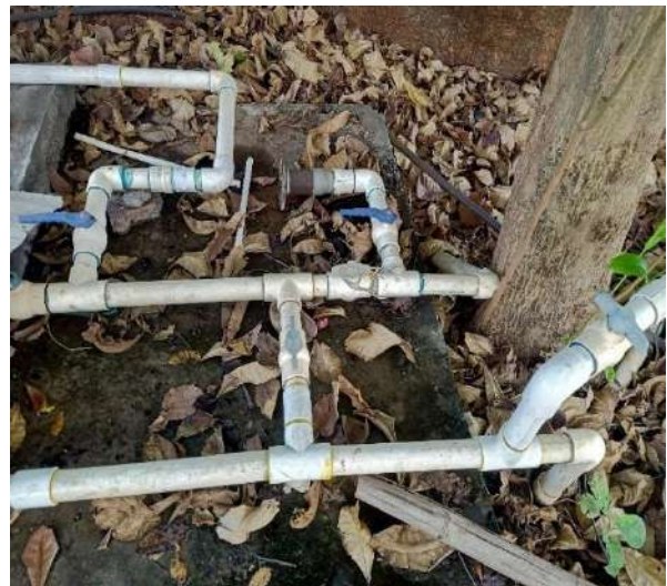
Plate 2. Water meter pipes to track consumption
