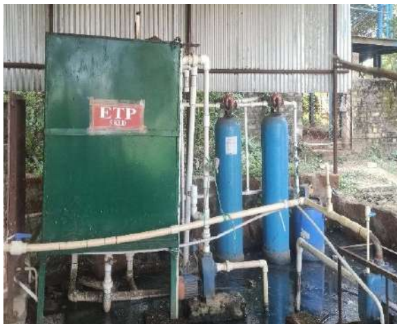
Plate 10. Effluent Treatment Plant
