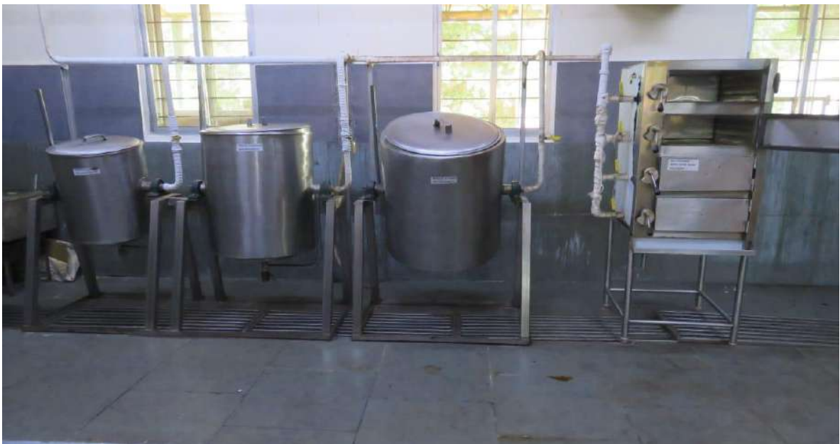
Plate 8. Steam boiler for kitchen in SSU
