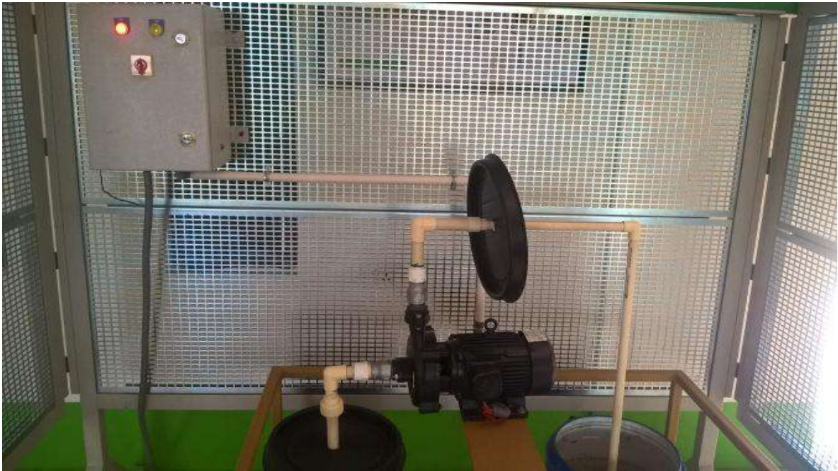
Plate 7. Solar water pump in SSU
