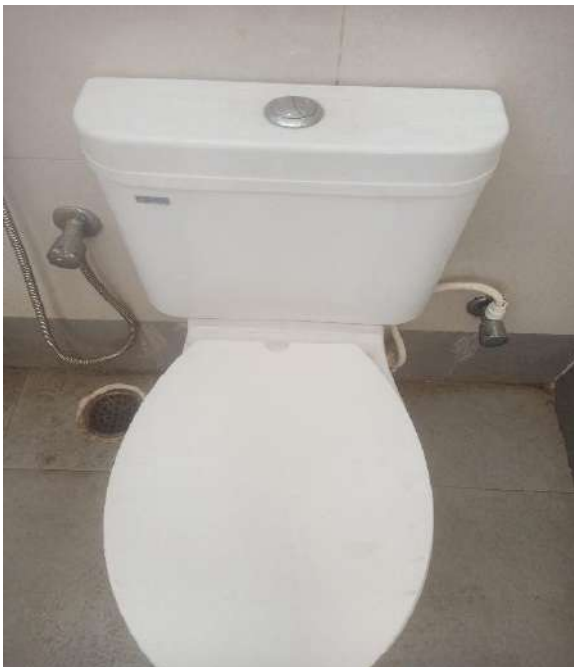
Plate 1. Dual flush toilets in SSU
