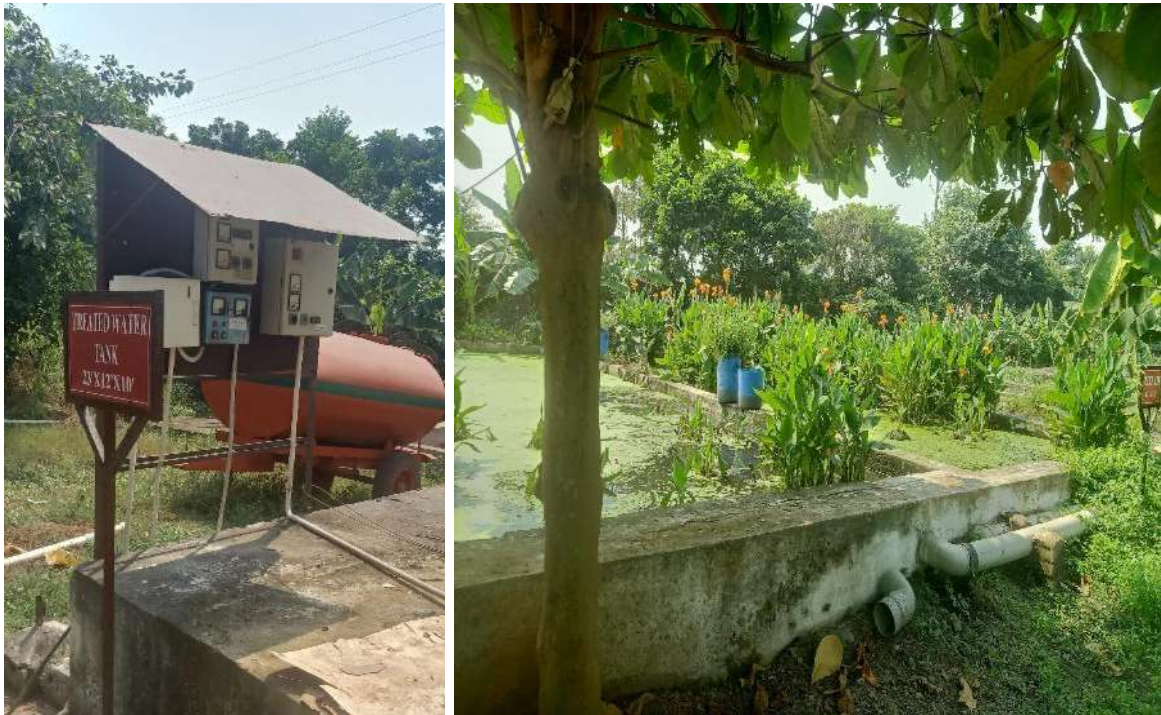
Plate 4. Biological Sewage Treatment Plant (Bio-STP) installed in SSU
