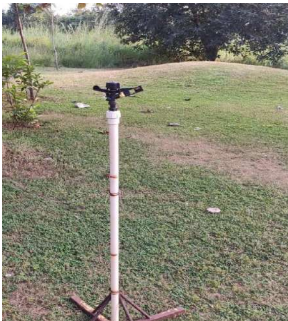
Plate 2. Sprinklers installed in SSU
