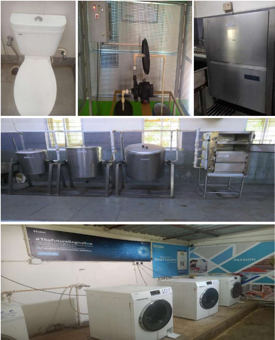
Plate 3. Water efficient appliances installed in SSU
