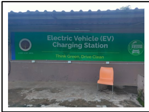
Plate 11 Electric Vehicle Charging Station
