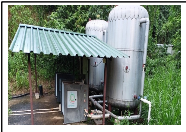
Plate 7 Air Sourced Water Heater
