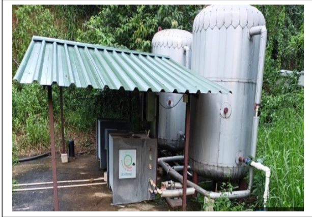
Plate 7.2.4.f. Air sourced water heater
