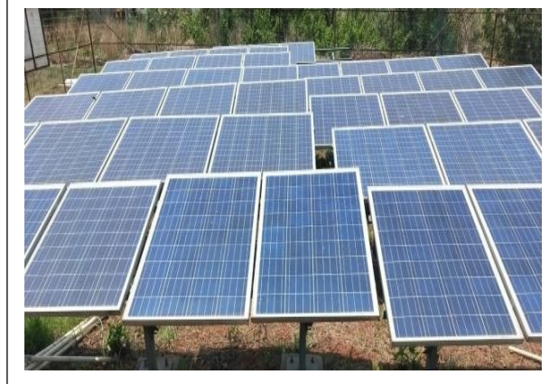
Plate 7.2.4.b 8kW Solar panel
