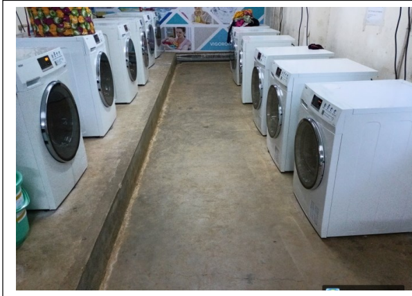
Plate 7.2.4.e. Centralized IOT based Washing Machine
