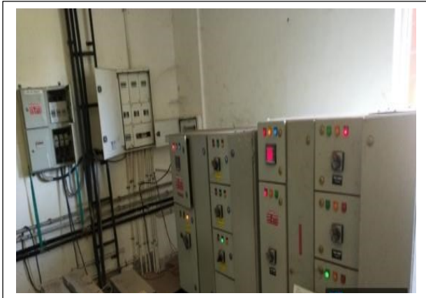
Plate 7.2.4.c. Electric control room
