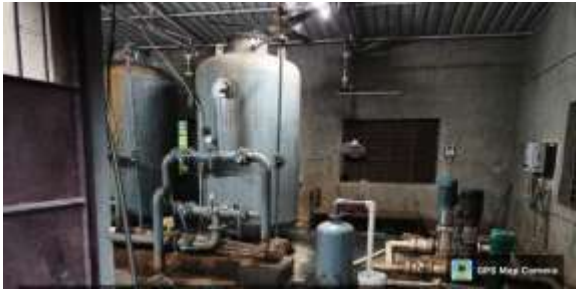
Plate 5. Drinking water treatment plant
