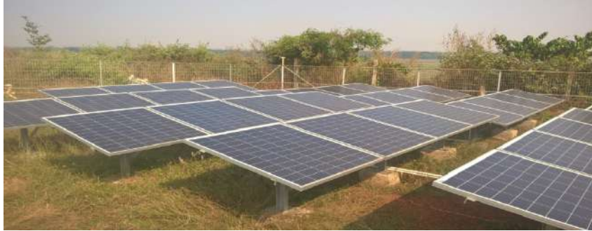
Plate 7. Solar Panel in University campus
