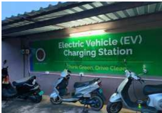
Plate 8. Charging station of e-vehicles
