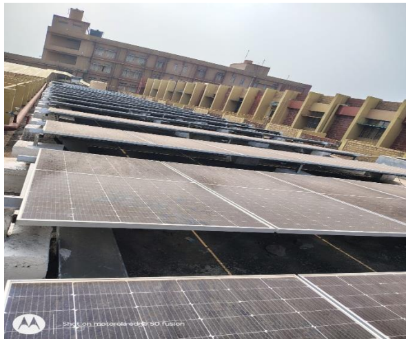
Plate 1. Roof top solar panel
