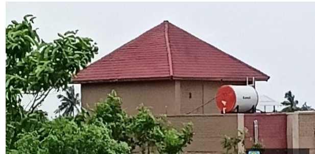
Plate 2. Rooftop solar heater
