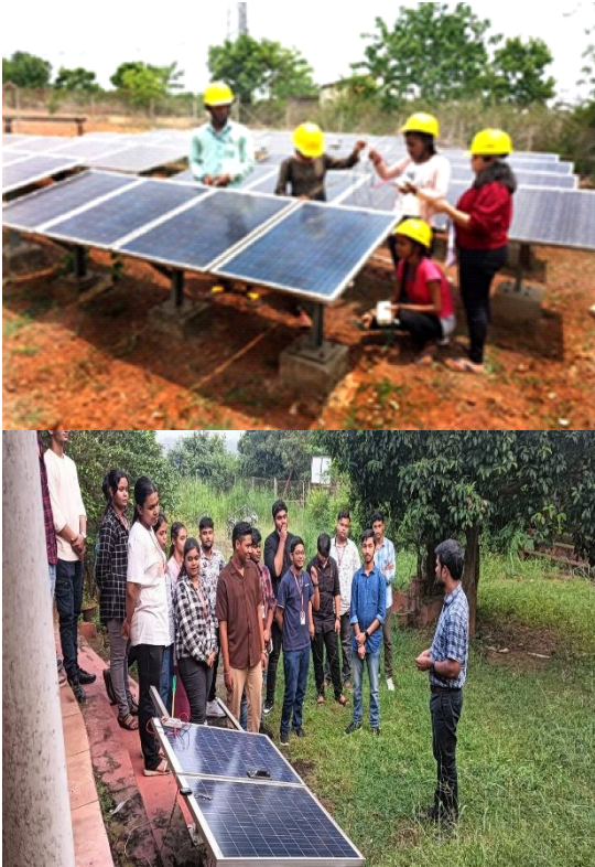
Plate 2. 8 Kw solar panels installed initially on the campus
