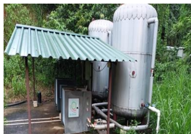
Plate 7 Air Sourced Water Heater
