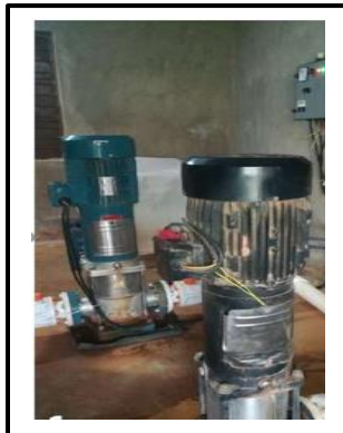
Plate 4 ground water pump
