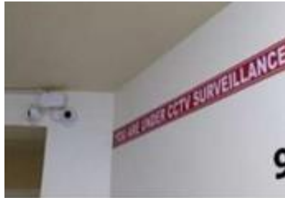
Plate 17. 24-hour CCTV surveillance
