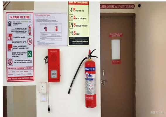
Plate 19. Fire alarm system
