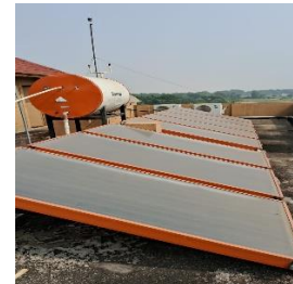
Plate 9 Solar Water Heater
