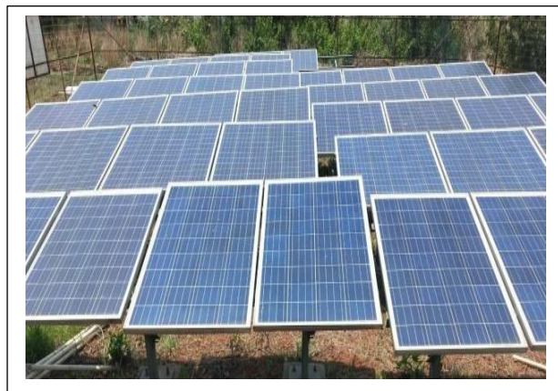
Plate 7.2.4b 8kW Solar panel
