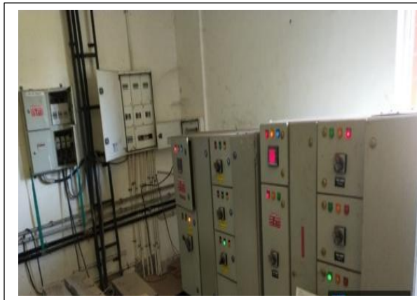
Plate 7.2.4c. Electric control room
